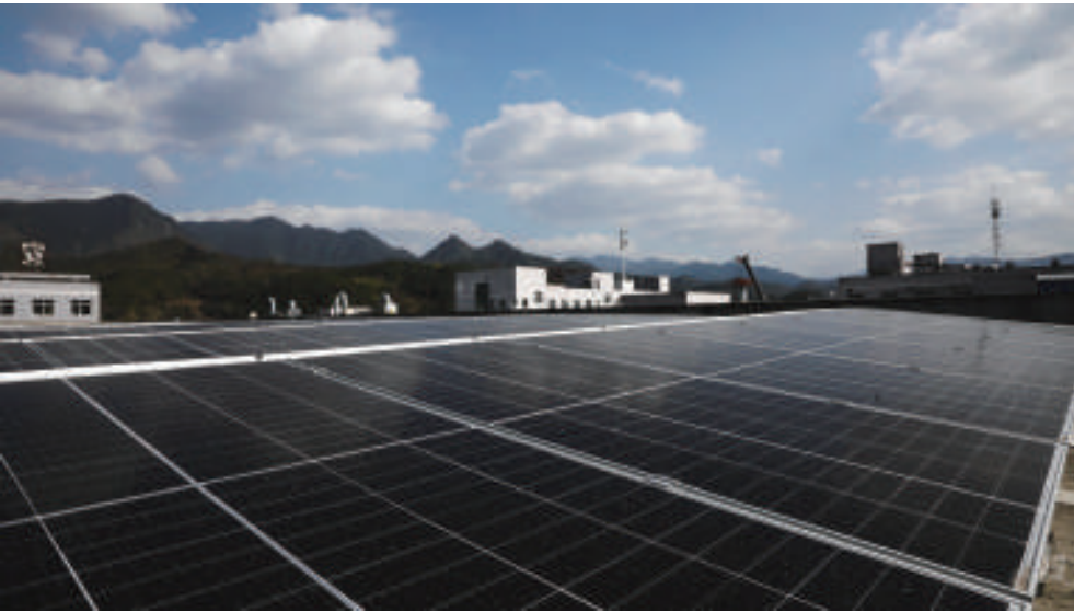
Qingtian County, Lishui, Zhejiang Province 400kW Vertex industrial/commercial distributed power project
