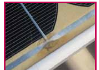
Yellowing and corroding panel
