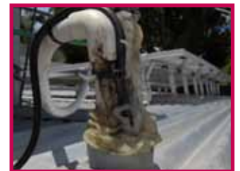
Poor installation quality
